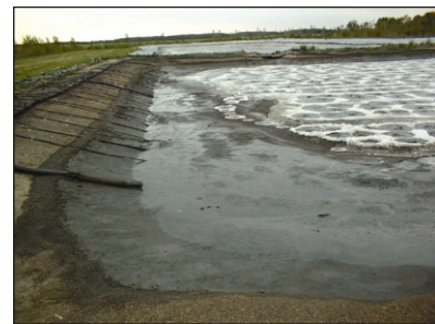
Figure 5. Air agitation of manure through piping system on storage bottom. Photo courtesy DGH Engineering.
