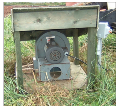
Figure 3. Centrifugal fan supplying negative pressure.
